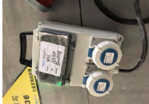
Electricity box of venue
